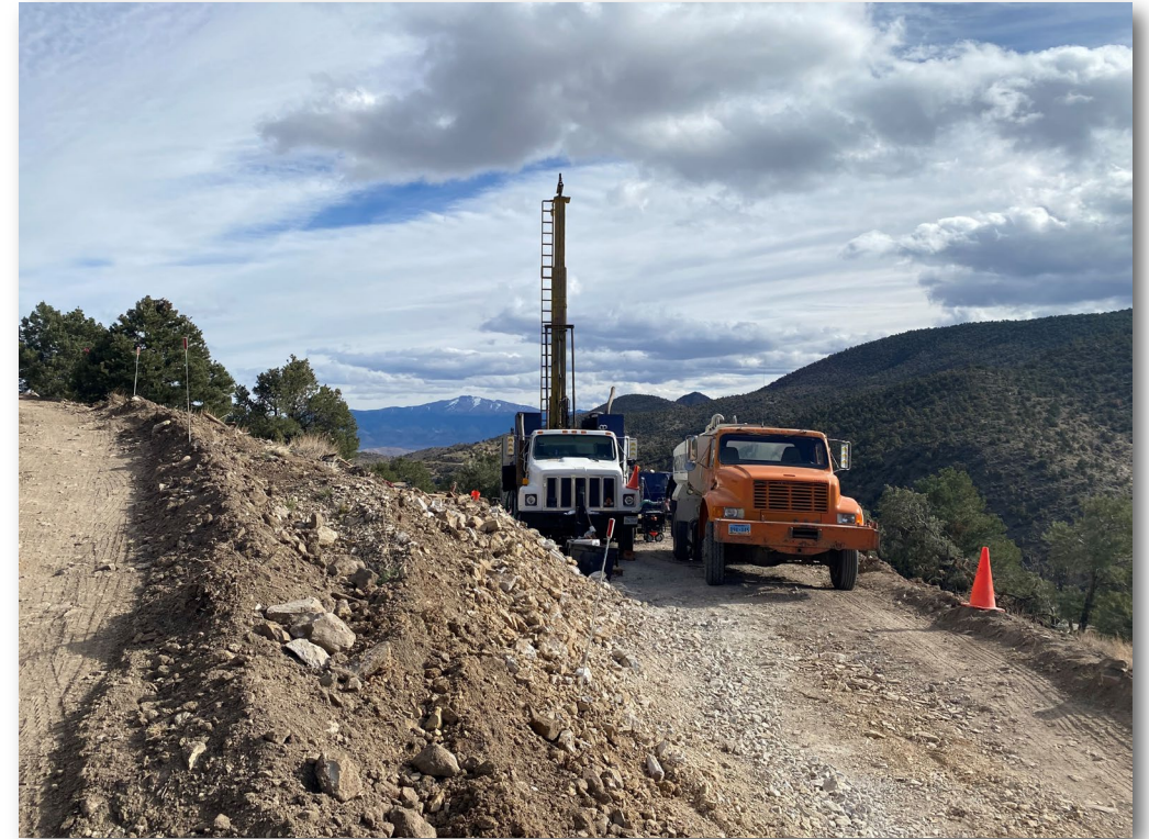
Drilling on Wilson Deposit with a view of the Wheeler Deposit in the background.
